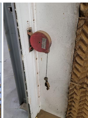
Ground cable - CFS Paint Booth
