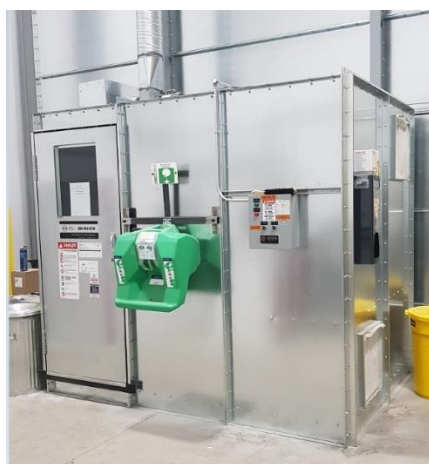
CFS Paint Booth – Mixing/Cleaning Room
