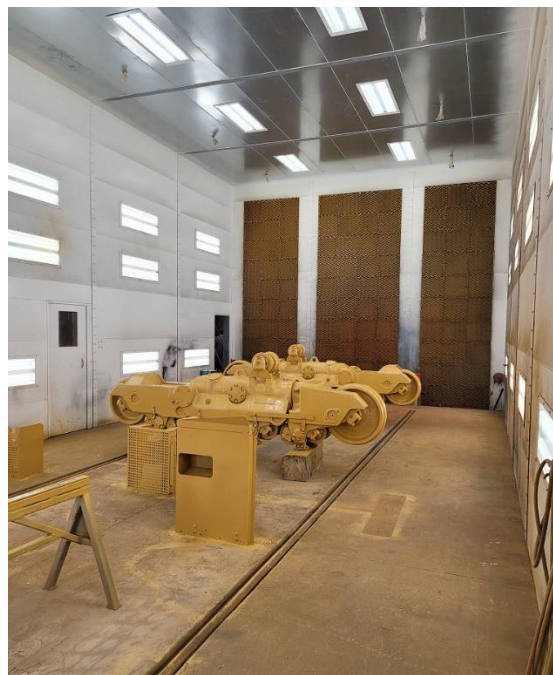
CFS Paint Booth
