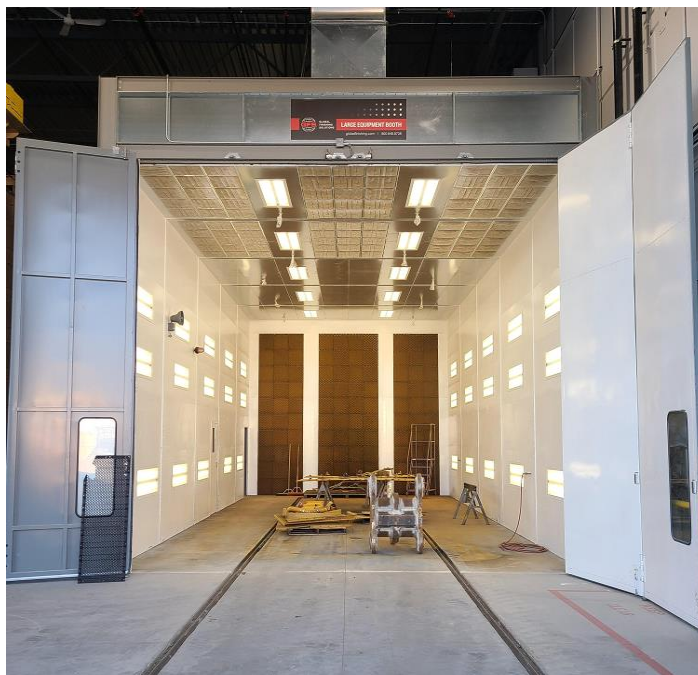
CFS Paint Booth
