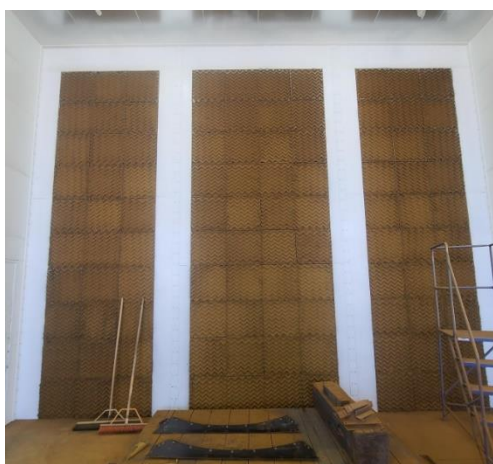
CFS Paint Booth – Filter System
